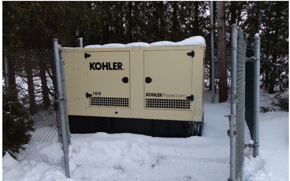
A KOHLER 100REOZJF provides emergency standby power for the sewer system in Jay, Vermont.
